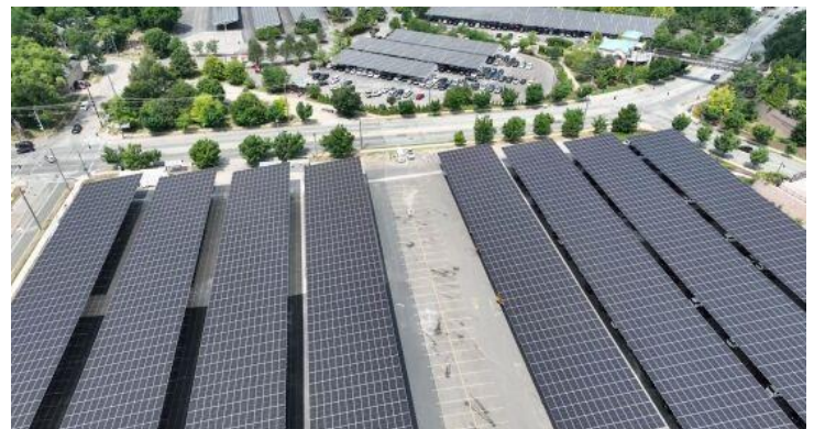
Source: Cincinnati Zoo, 2024, New Solar Array Over Second Parking Lot at Cincinnati Zoo Pumps Out Power and Provides Shade for Cars -
